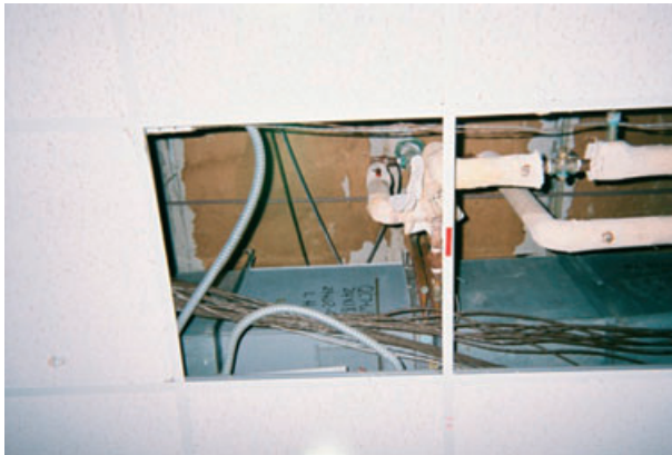
Figure 10. A missing acoustic tile in the ceiling may influence sense of self.
